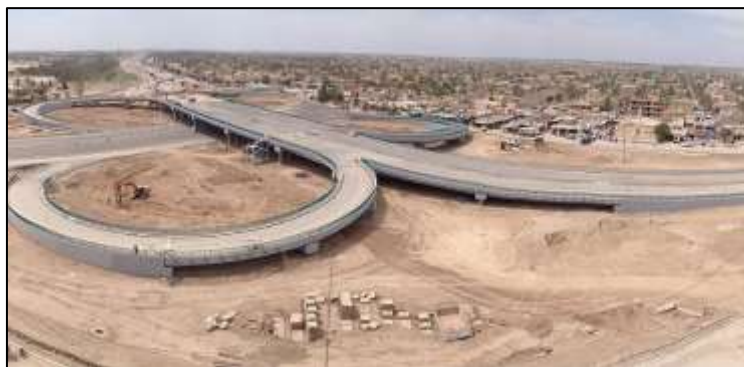
Figure 1. The case study area of the AL-Mafraq bridge at Baquba–Almafraaq region in Diyala Governorate.
