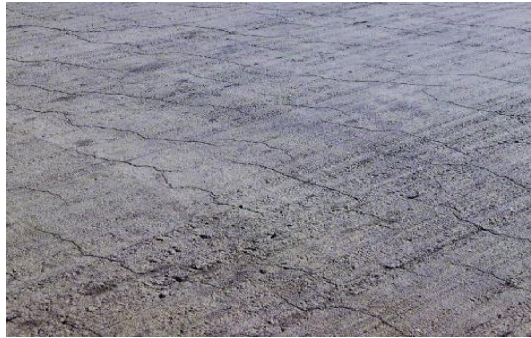
Figure 1. Plastic shrinkage on the concrete surface (Sayahi, 2019) .
