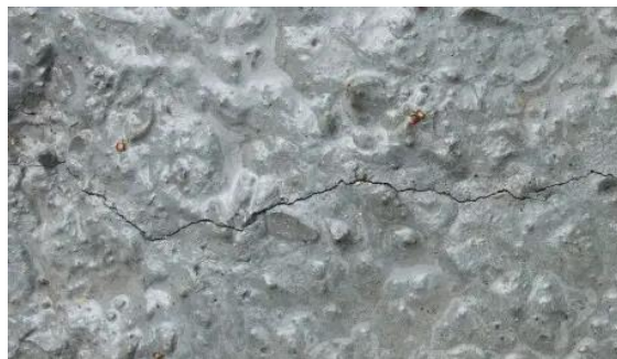
Figure 2. Dry shrinkage in the cemented concrete surface (Safiuddin et al., 2018) .
